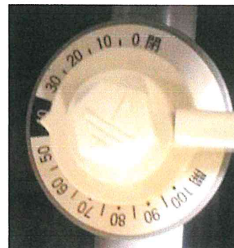
At start-up, and for standard operation, the Effluent Airlift Valve (white) should be set to 40%. 18
