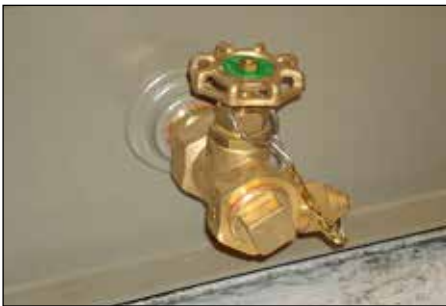
Figure 3. Drain valve with sampler.
