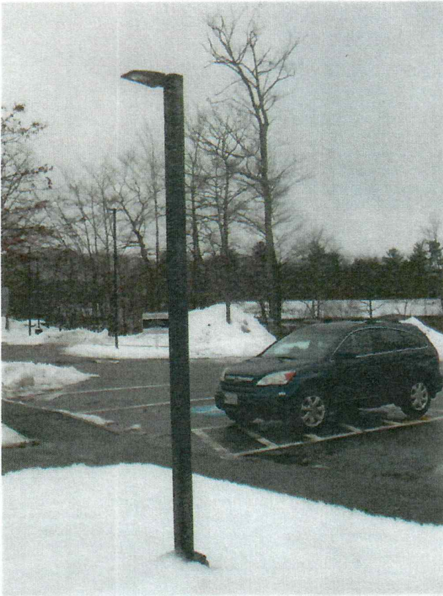
Parking Lot Lighting
