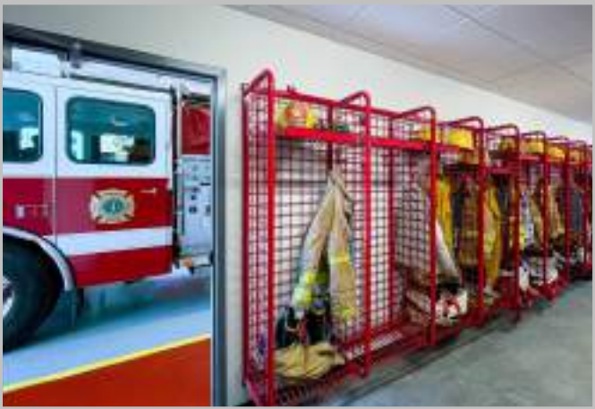
Turn Out Gear Room
