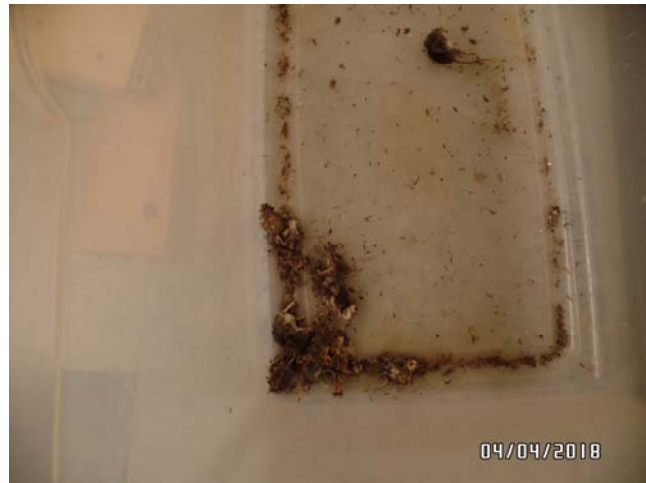
Evidence of animal/rodent activity. Feces were observed above drop ceiling areas.
