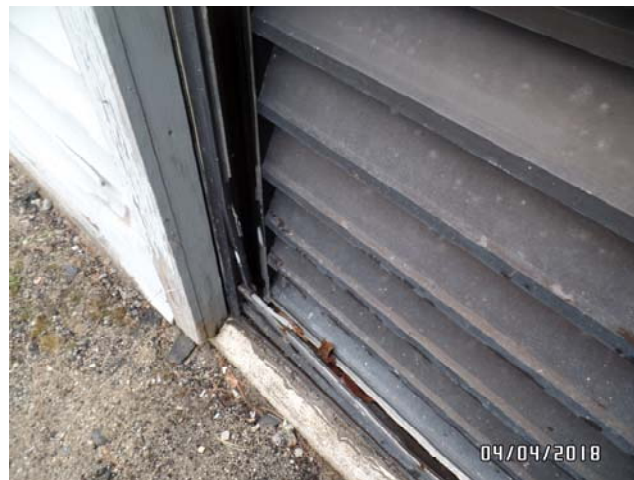
Damaged ventilation grate is easy access to wall cavity for small rodents.
