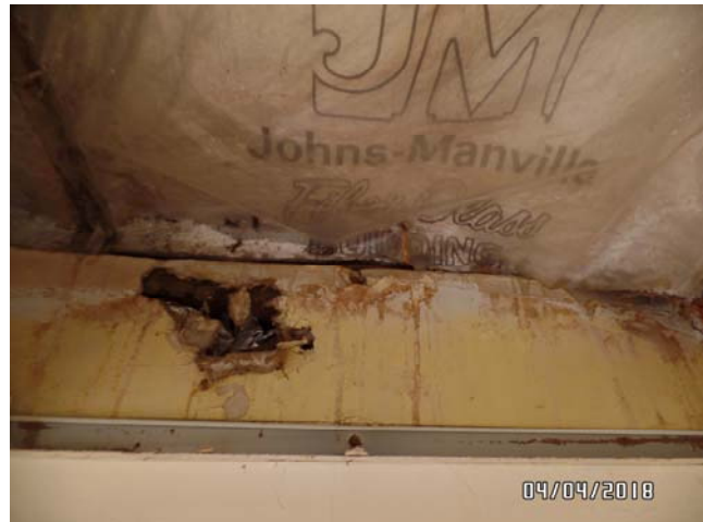
Water damaged drywall above drop ceiling area.
