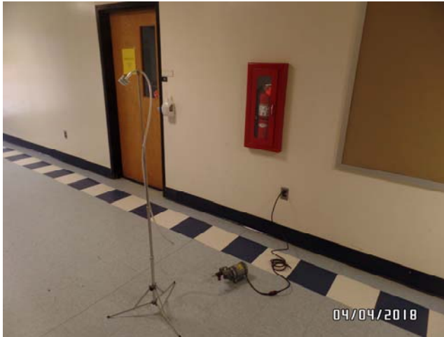
Mold Air Sample (A-7) in corridor near Room #19.
