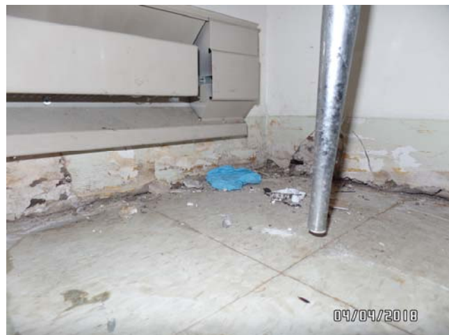
Lower drywall damage from previous water incident in Storage Room.
