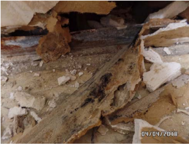
Visible mold growth in Storage Room lower wall.
