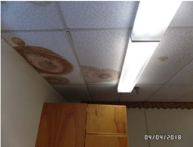
Stained ceiling were observed throughout building.
