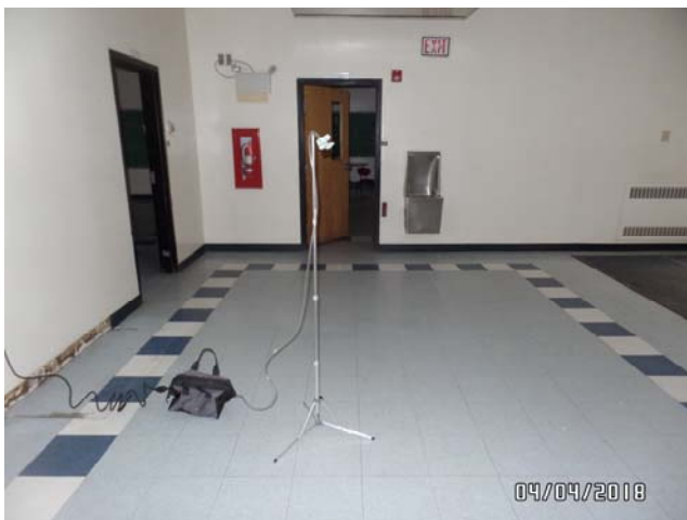
Mold Air Sample (A-5) in corridor near Room #14.
