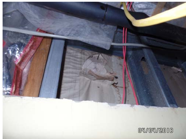
Water damaged drywall above drop ceiling area.
