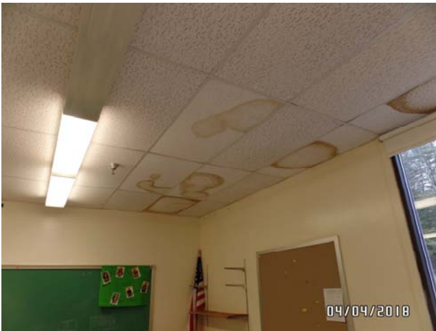
Stained ceiling were observed throughout building.
