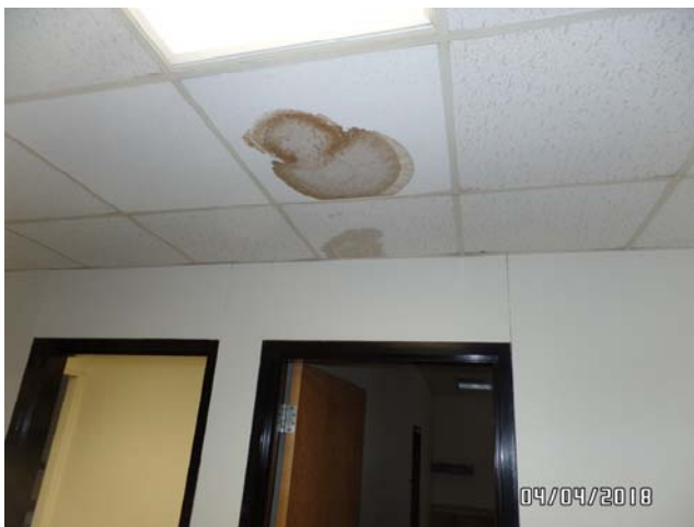
Stained ceiling were observed throughout building.
