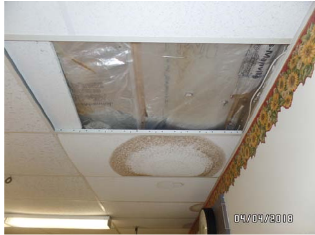
Stained ceiling were observed throughout building.
