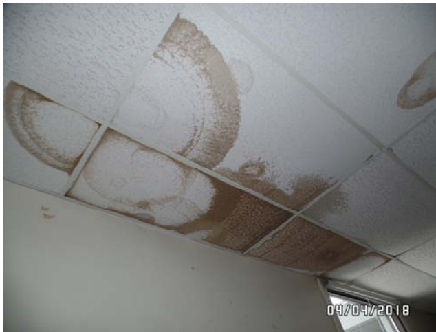
Stained ceiling were observed throughout building.
