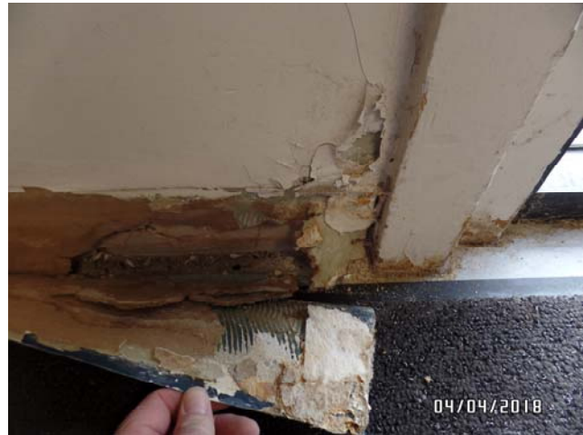
Water damage to lower drywall around entry doorways.
