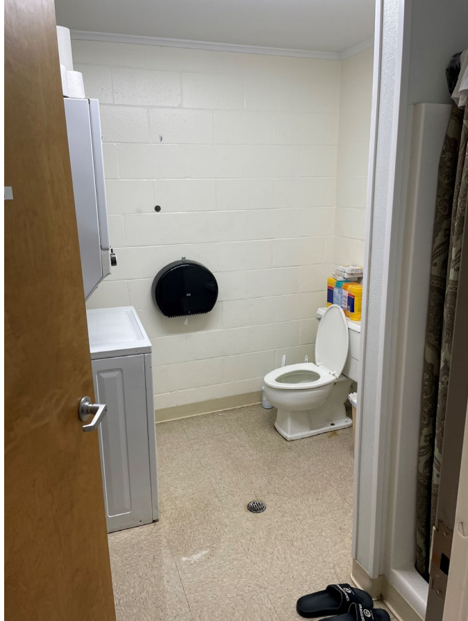
Non-compliant ADA bathroom
