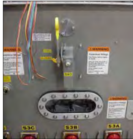
Figure 8. VFI transformer with visible break.
