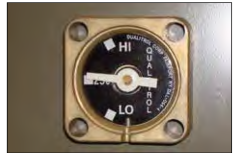
Figure 5. Liquid level gauge.
