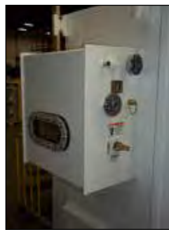
Figure 7. External visible break with gauges.
